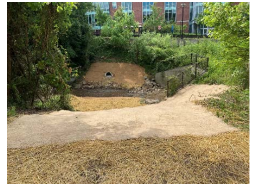
Repaired stormwater outfall and restored channel adjacent to the Townsontown Parking Garage.
