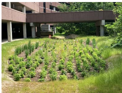
Townsontown Parking Garage bioretention facility post-construction. Ecotone crews addressed erosion issues, removed sediment, and installed plantings.
