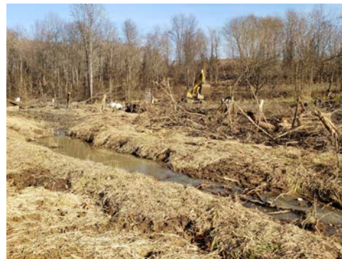
During construction, the crews incorporated woody material and a roughness approach to grading to add micro-topography and enhance habitat in the floodplain.
