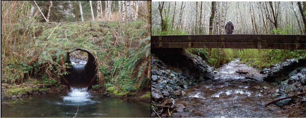
Figure 1. Undersized Culvert and Bridge Replacement
