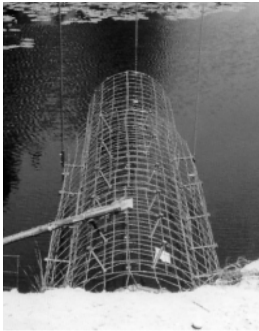
Figure 3. An installed Beaver Stop. (Photo courtesy of FSI Culvert Inc.)
